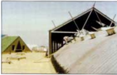
BUR system at The Promenade in Temecula in Temecula, California, showing flashing prior to installation of OSB, rigid insulation substrate.
