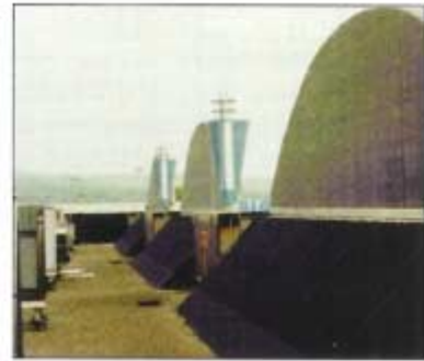
New parapet construction with an EPDM membrane on the vertical surface and new modified bituminous roofing on the existing sloped surface, with metal transition flashing between (Wayne Hills Mall, Wayne, New Jersey).
